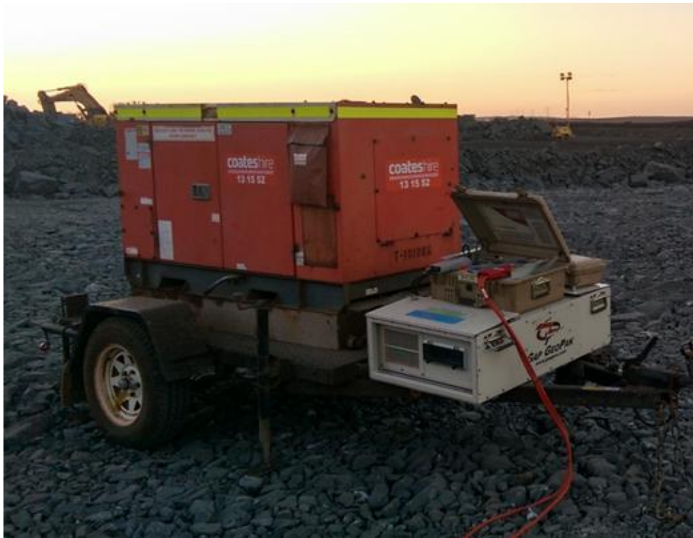
FIGURE 8. FIXED LOOP TRANSMITTER SYSTEM. EODTX200 TRANSMITTER POWERED BY PS10LV AND 3-PHASE GENERATOR.
